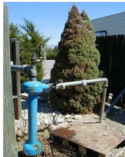
Figure 1: The wellhead on your property will typically include a pipe leading to your pressure tank.
