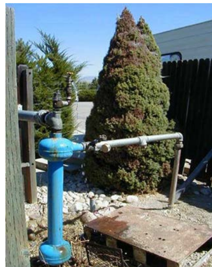
Figure 1: The wellhead on your property will typically include a pipe leading to your pressure tank.
